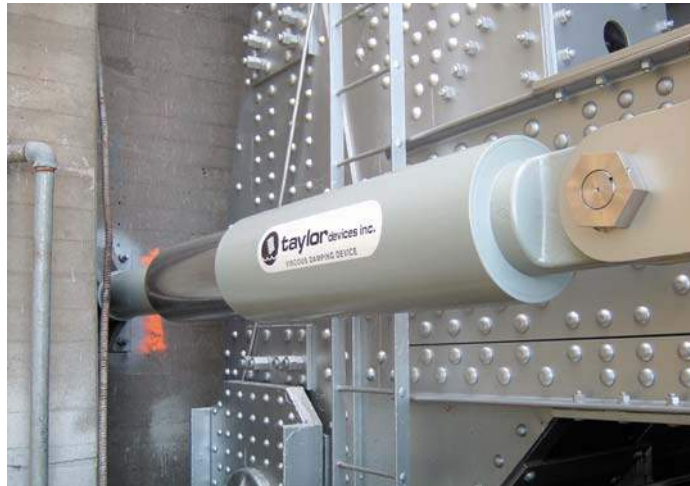
Seismic damper installed where the western portion (suspension spans) of the San Francisco-Oakland Bay Bridge meets Yerba Buena Island
